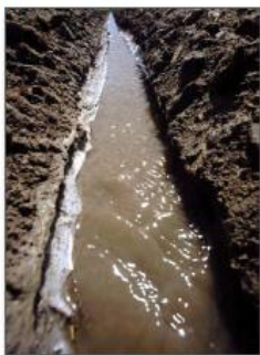
Figure 23. Untreated furrow with erosion
