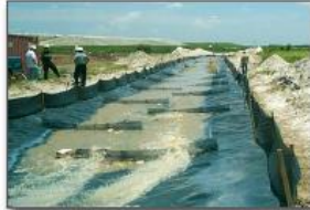
Figure 16. Flocculation ditch with checks to increase the polymer mixing
