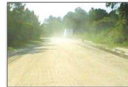
Figure 12. Road dust before applying polymer flocculant
