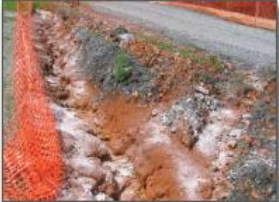
Figure 38. Eroding gully on a construction site
