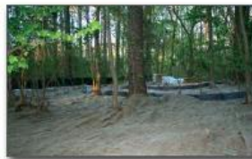
Figure 9. Dispersion field with jute matting and flocculant powder
