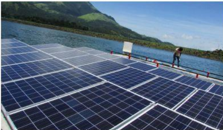
10kW Floating Solar Power Plant installed in Banasurasagar
