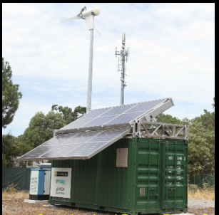
Curtin Uni containerized solar-hybrid power system
